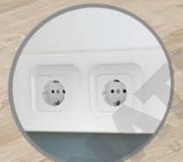
Hidden Power Sockets
